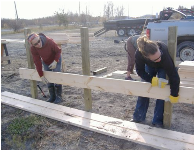
Installing part of the soil retaining wall at the Old Town garden site.
